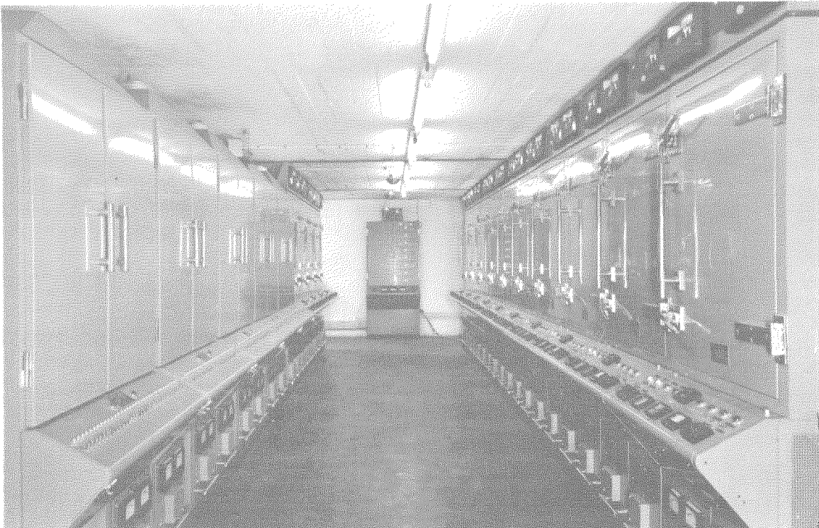
Figure 9—In this room 19 temperature-stabilized ovens are used to test components in extreme environmental conditions.
